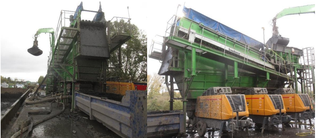
Starscreen with 1.7 m screen width as a protective screen for a sewer excavation feed pump. Screening is implemented at a diameter of 60 mm and a maximum length of 180 mm. The fine fraction is delivered 500 - 800 m by 3 concrete pumps.
